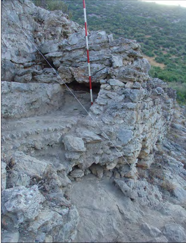
Fig. 12: Hadrian aqueduct with stone slab covering and above a supporting pillar of the Antonine aqueduct in section XV.
